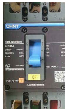
Figure 2.1-1 Lower electrical box breaker (break state)
